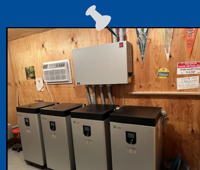
Photo 3: Battery Bank (SimpliPhi eVault Max Units) Our four battery units — the energy storage backbone that keeps our home powered even when the grid goes down.
