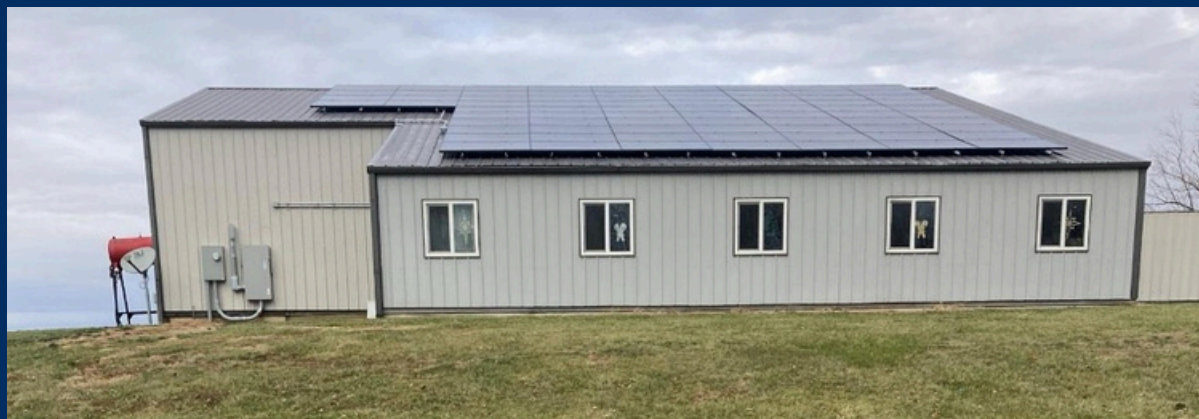
Photo 1: Solar Panels on the Barn Roof Our barn roof fully outfitted with 78 solar panels — the heart of our renewable energy system.
