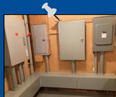
Photo 2: Electrical Service Wall The upgraded electrical service that ties our solar panels, inverters, and batteries into a seamless whole-home system.
