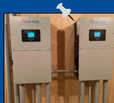
Photo 4: Dual Sol-Ark Inverters Our two Sol-Ark hybrid inverters — the brains of the system, converting solar energy into usable household power.
